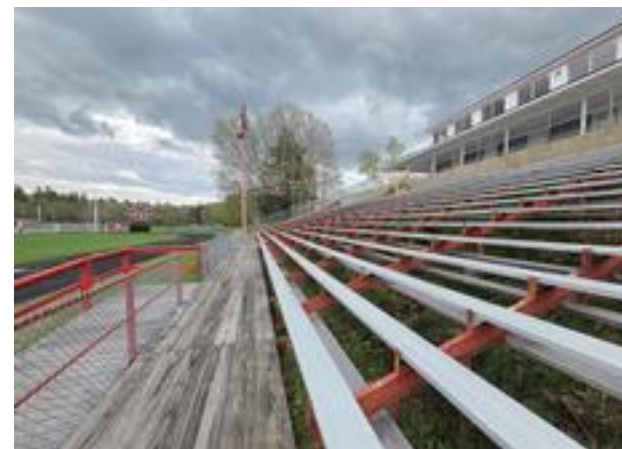
Bleachers at Cobb Stadium are too costly to repair, school officials say.
