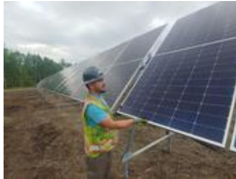
Dalton Enius of Solar Operation Solutions installs panels at the former CGA site off New Dam Road. Photo: Lee Burnett
