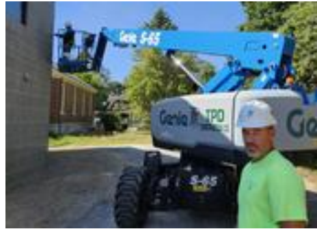
Greg Dumont, project supervisor for TPD Construction, eyes things on the ground while a masonry contractor gets a bird's eye view of Goodall Library's expansion.
