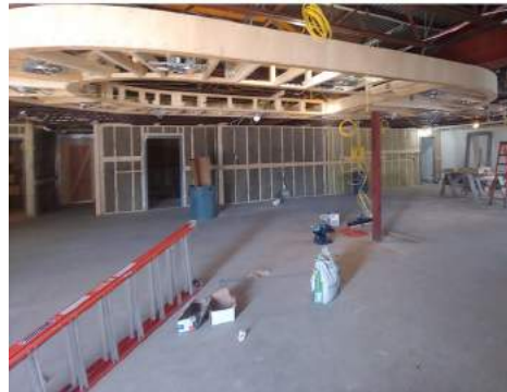
The interior of Goodall Library, showing the partially constructed circulation desk area. Photo: Lee Burnett
