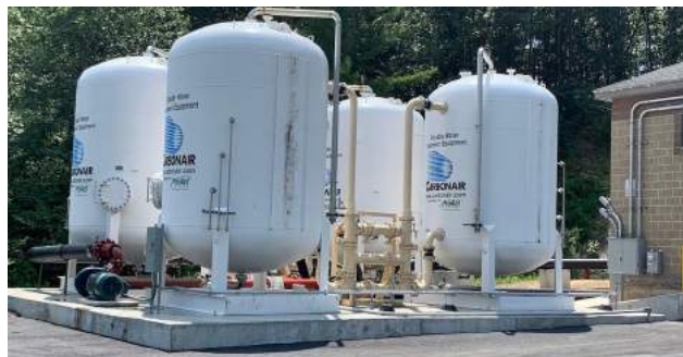
The Sanford Water District is exploring installation of an ion exchange water filtration technology, a more compact version of this treatment plant in Hudson Mass. Photo: Massachusetts Municipal Association
